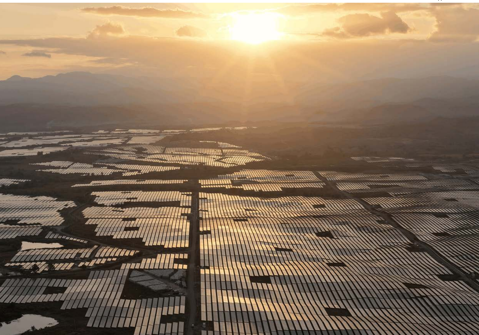
The MTerra project achieved initial grid synchronization in February 2026, just 15 months after its groundbreaking.
